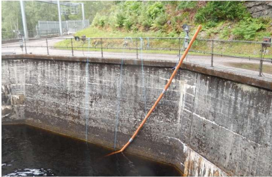
The fish introduction pipe at the intake, extending down to the submerged intake opening.
