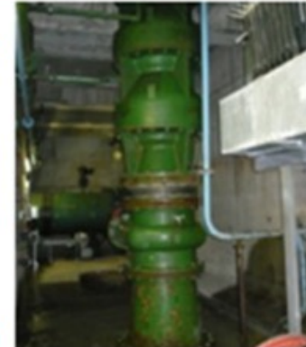
Fig 1. Existing pumps at Coppermills AWTW
